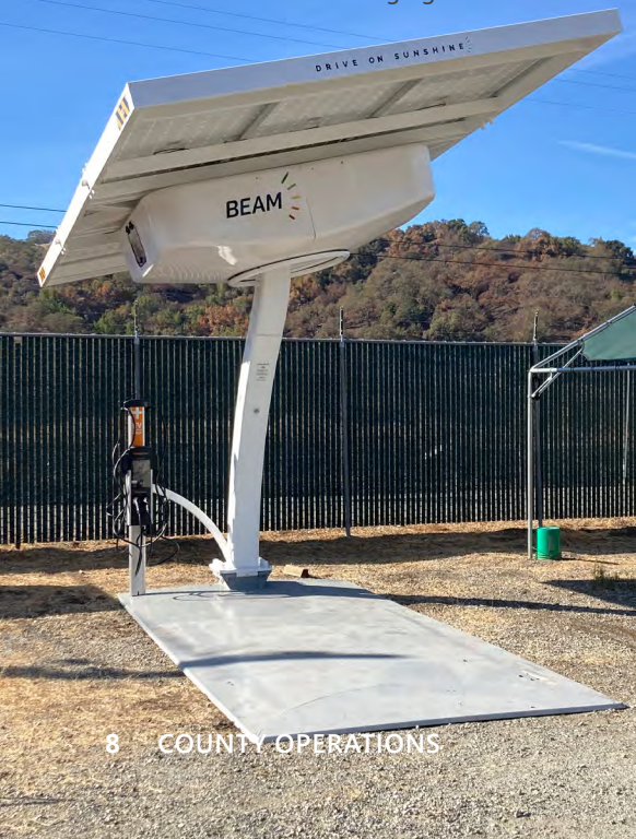
Parks Mobile EV Charging Unit
